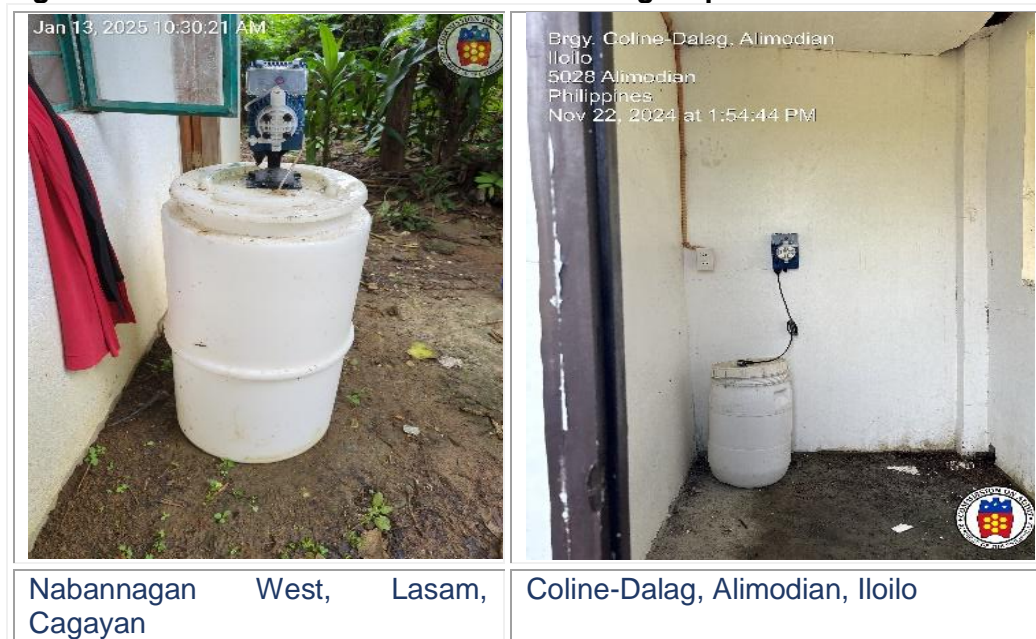
Figure 17: Non-Functional Chlorinators During Inspection
